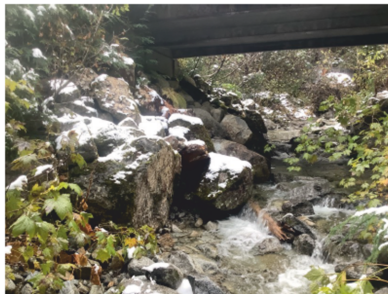
Downstream right riprap scour
